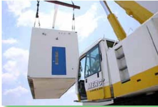
Figure 5 Portable classroom being lifted into place. Photo courtesy of Royal Concrete Concepts, Inc.
